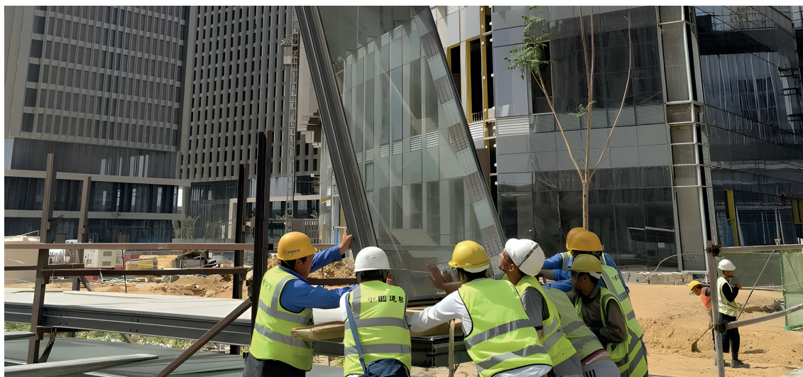
Chinese and Egyptian workers are working together on the construction of the new capital, which is not only a key project of the Belt and Road Initiative but also the largest project Chinese companies are building in Egypt (Photo: Xinhua, 2023).
