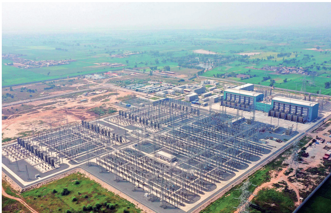
The Lahore Converter Station is part of the CPEC high-voltage direct current transmission line project located in the eastern Punjab Province of Pakistan (Photo: Xinhua, 2022).
