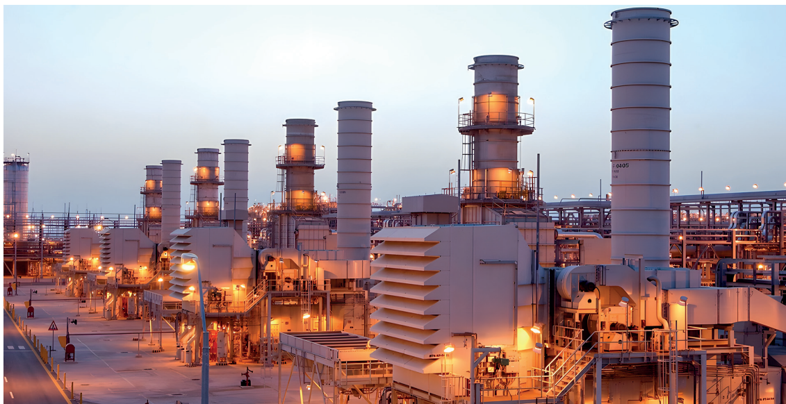
Yanbu Aramco Sinopec Refining Company (YASREF), a joint venture between Saudi Aramco and China Petrochemical Corporation (Sinopec), is China's largest investment project in Saudi Arabia (Photo: CGTN,2023).
