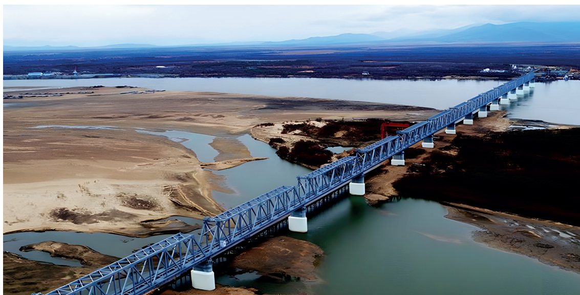
Photo taken on April 26, 2017 shows the China-Russia Tongjiang-Nizhneleninskoye railway bridge under construction as part of the Belt and Road Initiative (Photo: Xinhua, 2018).
