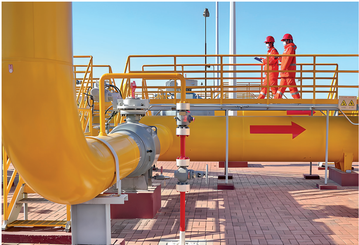
November 2022, during inspection work on the China-Russia eastern route natural gas pipeline in Qinhuangdao, northern China's Hebei Province (Photo: CGTN, 2022).
