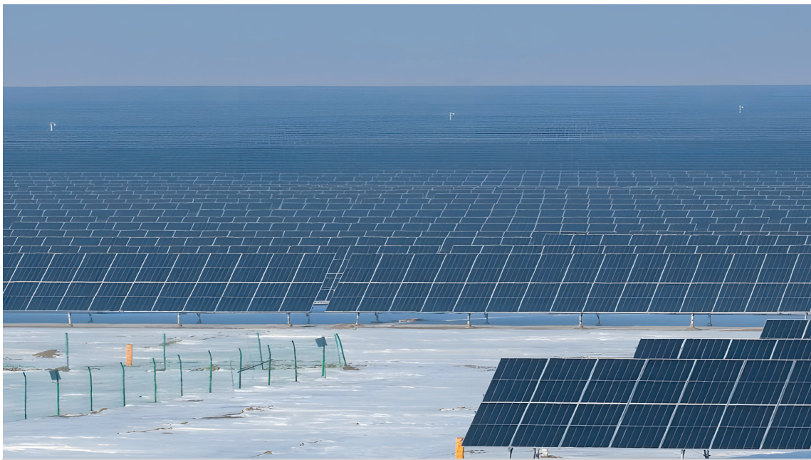
A photovoltaic power project in Kazak Autonomous County of Mori, Changji Hui Autonomous Prefecture, northwest China's Xinjiang Uygur Autonomous Region, December 20, 2023 (Photograph: Xinhua, 2023).
