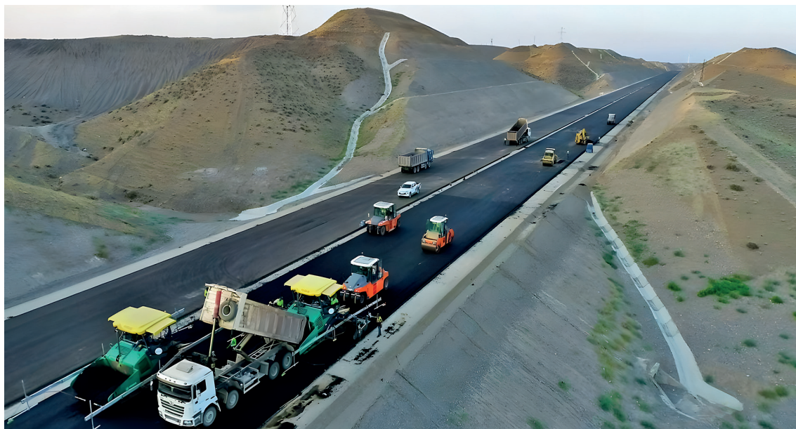
A frame from the construction phase of the Zengezur Corridor, an important initiative for transportation between Turkic States (Photo: Aayda, 2022).
